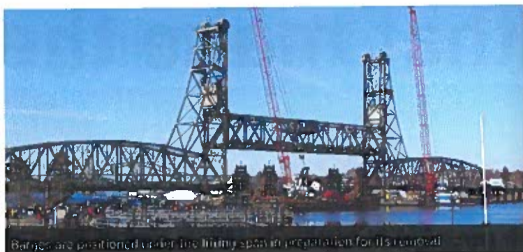
Barges are positioned under the lifting span in preparation for its removal
